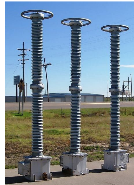
Capacitive Voltage Transformer (CVT)
